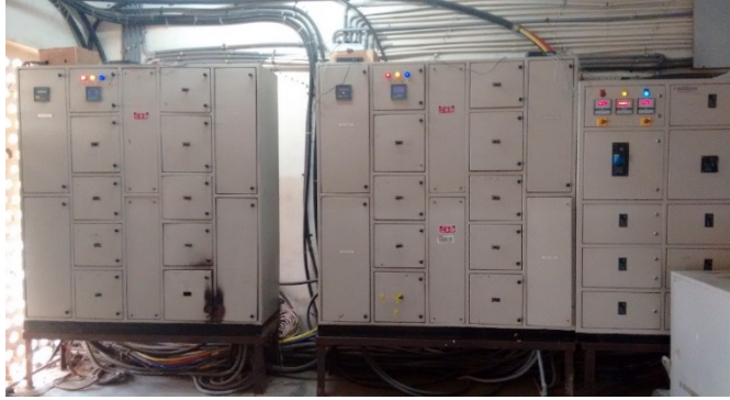
Meter deployment at Electrical Panels-1
