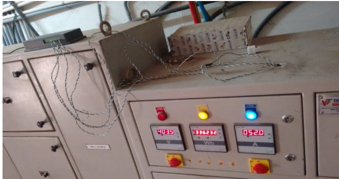
Meter deployment at Electrical Panels-3
