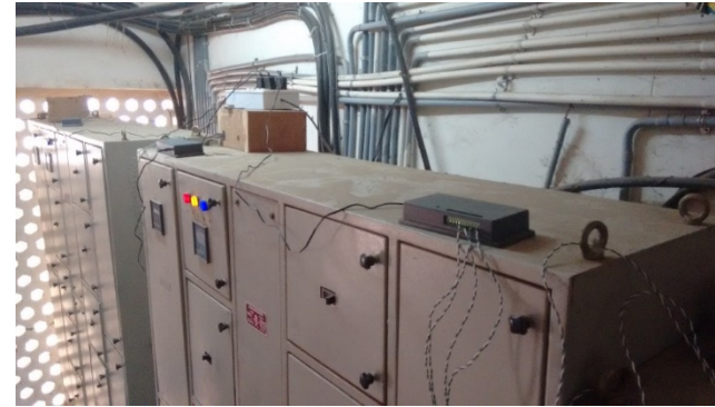
Meter deployment at Electrical Panels-2
